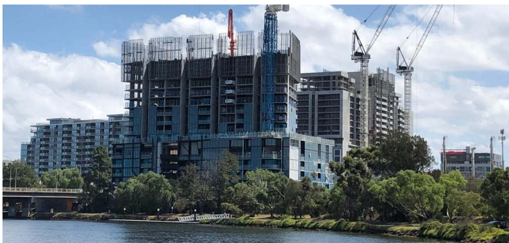
Figure 3 Joseph Road Precinct development activity viewed from Maribyrnong River and river walkway reserve
